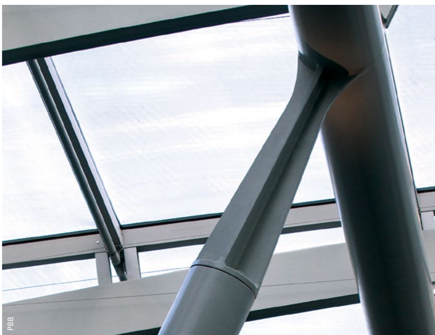
ABOVE: Columns and rafters incorporate XLERPLATE® steel made by BlueScope. The laser-cut and hand-welded steel achieves a beautifully detailed edge
